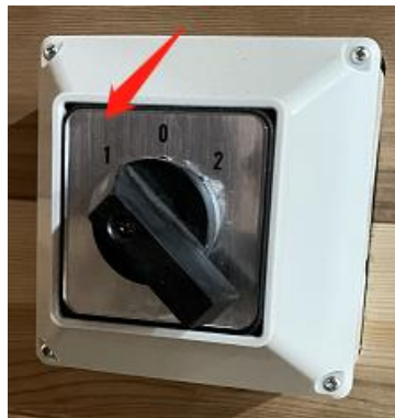
Power to stove heater
