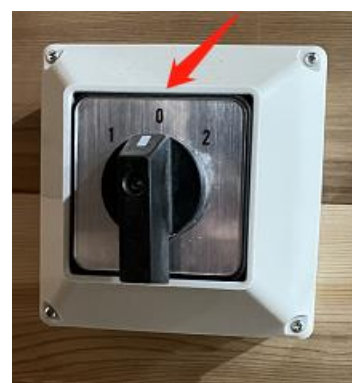
Power turned OFF
