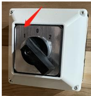
Power to stove heater
