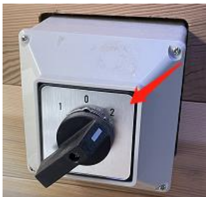
Power to Infrared heaters
